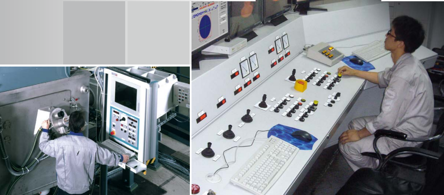
Local operation panels
